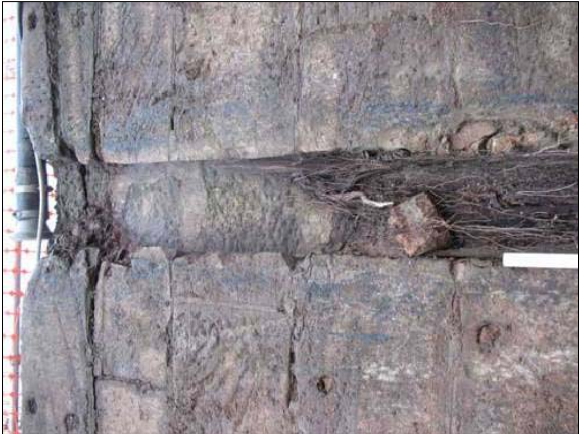
Figure 7a: Detail showing Vertical Slot Cut into Masonry of Outer Face, Inner Wall
