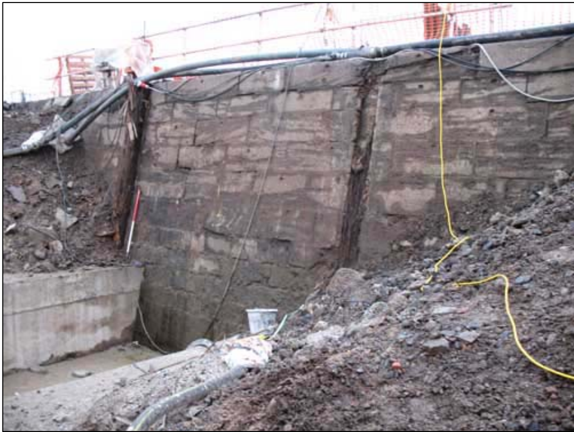
Figure 6a: Outer Face of Inner Harbour Wall, With In Situ Timber to left
